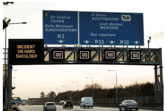
Completed gantry with ITS equipment.
