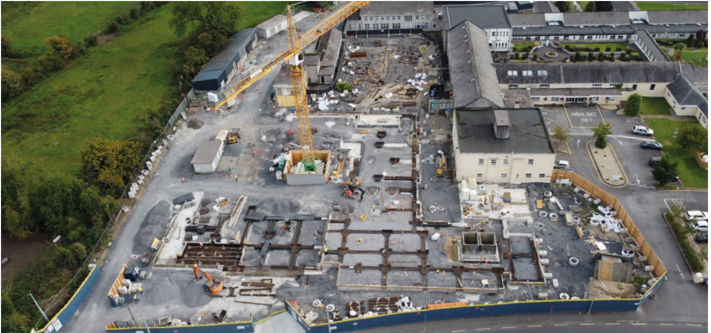
An aerial view of the building under construction. Image courtesy of Duggan Brothers Ltd.
