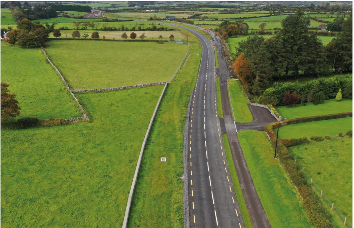
Aerial view of the ongoing works along the N60 showing the integration of an active travel facility alongside the realigned Type 2 single carriageway.
